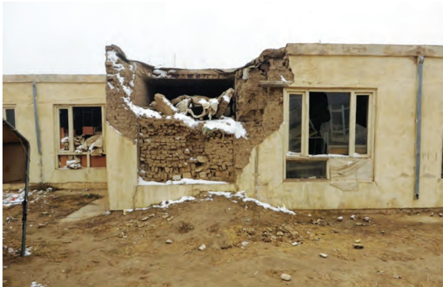
The wall and roof of a school in Baghlan Province that was damaged by an explosion. (SIGAR photo)
