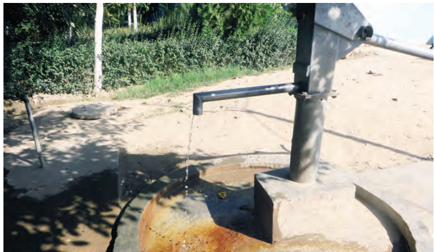
A functioning well at a school in Kunduz City. (SIGAR photo)
