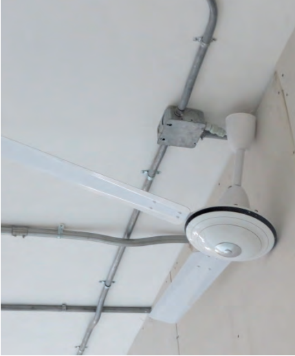
A suboptimal ceiling-fan installation at the Ministry of Interior headquarters building. (SIGAR photo)
