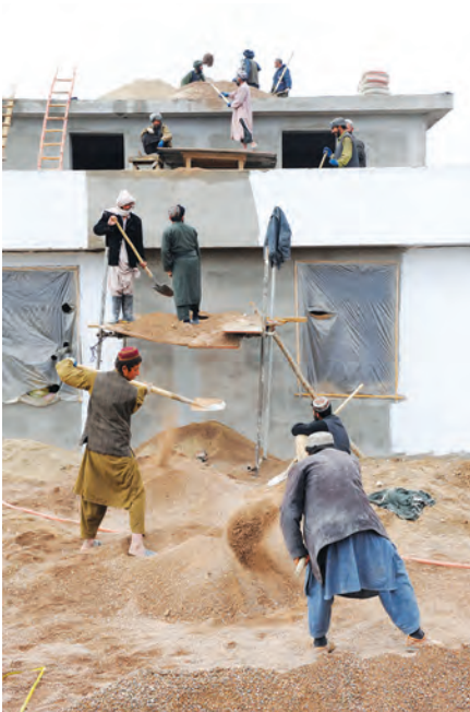
Workers move gravel up to the roof of a new prison in Uruzgan Province, 2011. (USAF photo by 1st Lt. Matt Schroff)
