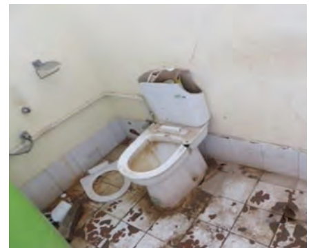
Broken toilet in the guard quarters building of Wardak Prison. (SIGAR photo)
